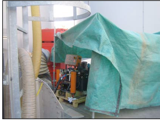
Covering and heating material
